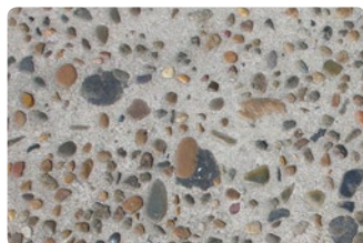
Exposed concrete aggregate
