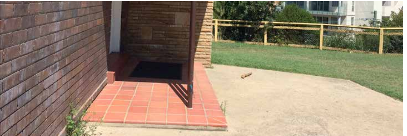
Image: no accessible entry to community building
