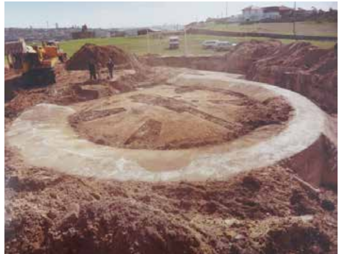
Image: Partially uncovered Ben Buckler gun emplacement in Hugh Bamford Reserve, October 1984.
