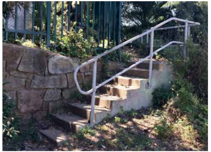
Image: Existing stairs are not compliant
