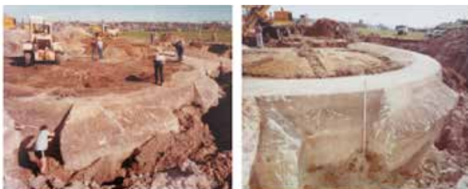
Images of the excavation of the Ben Buckler gun battery by Sydney Water in 1984 (Source GML Heritage Review 2019)
